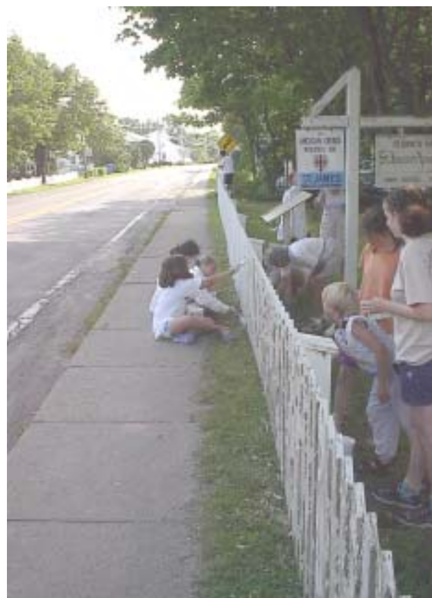
Two St James's churches get a little paint. Summer is short but it is also the time for repairs and repainting. St James, Lac Beauport, put out a call in the Quebec Chronicle-Telegraph in July in the hope of getting half a dozen volunteers to help repaint the church. According to lay reader Gayl Loosli "All the members of our congregation are pretty elderly" and so they need some outside help. Meanwhile at St James, Cacouna, children and grandchildren, pictured above, were coaxed into scragging, priming and painting the fence.
